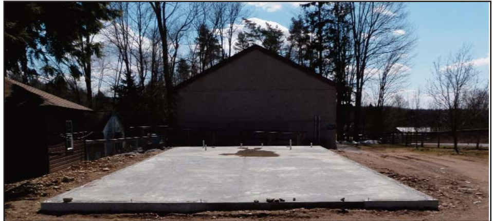
The concrete slab is ready for the new Arts & Crafts Building at Kamp Kiwanis. The old building is at left; in the background is the Morgenroth Drama Center.
